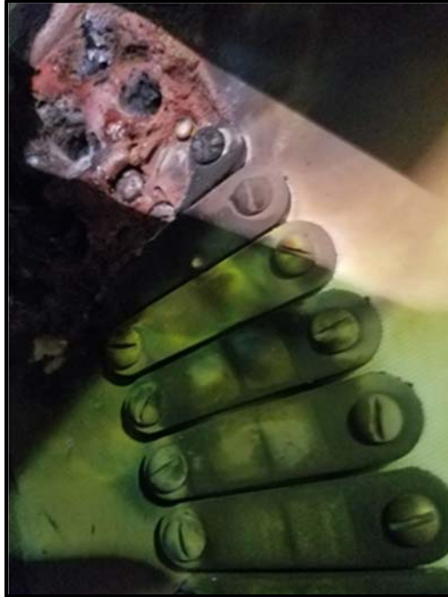
Figure 19 Field Rheostat Damage August 9, 2017
