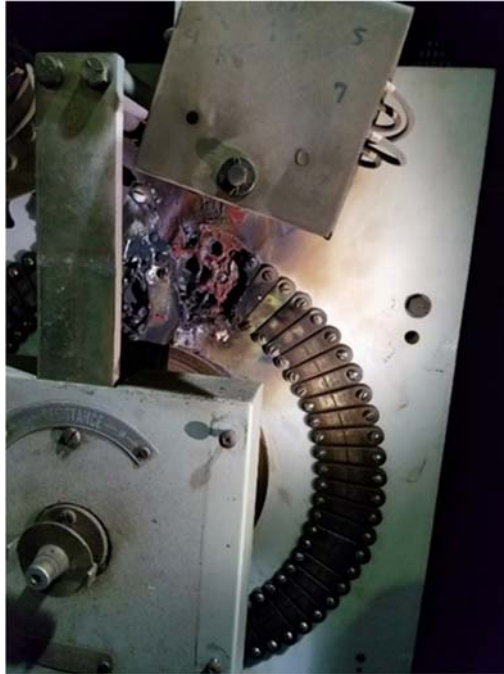
Figure 16 Damage to Field Rheostat
